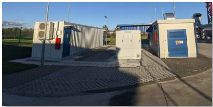
Veolia Gas Power Plant Levice, Slovakia Secondary Frequency Control System energy: 5.2 MW / 2.9 MWh
